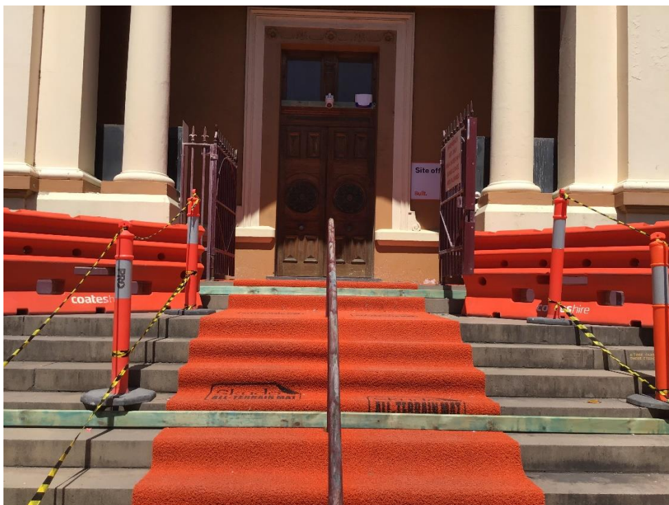
Photo 08: View of Main Entry to Courthouse. Note protection measures and CCTV camera & alarm mounted above the doorway.
